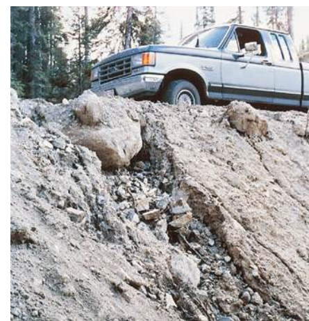
Soil sloughing off a road cut.
